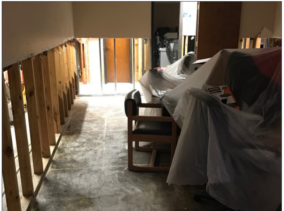
Hurricane Harvey flood damage at a TDCJ parole office.
